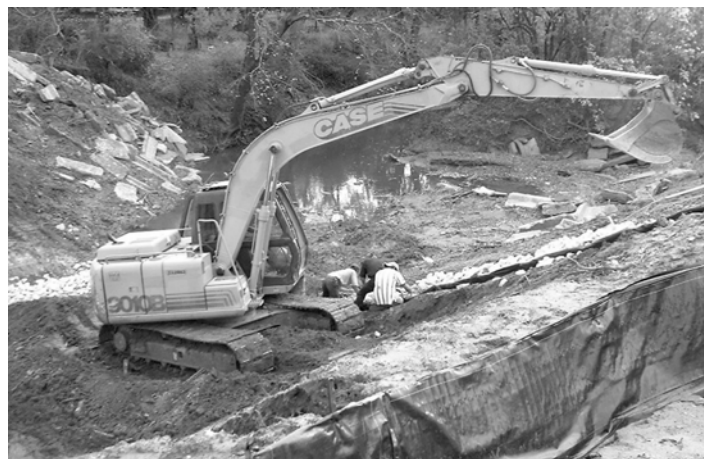
A sewer line crosses Johnson Creek near Mitchell and Pecan streets. Its route was changed to avoid nearby woods.
